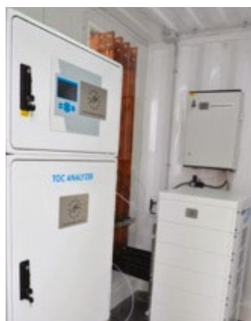
Figure 3: BioTector B7000 installed at the plant
